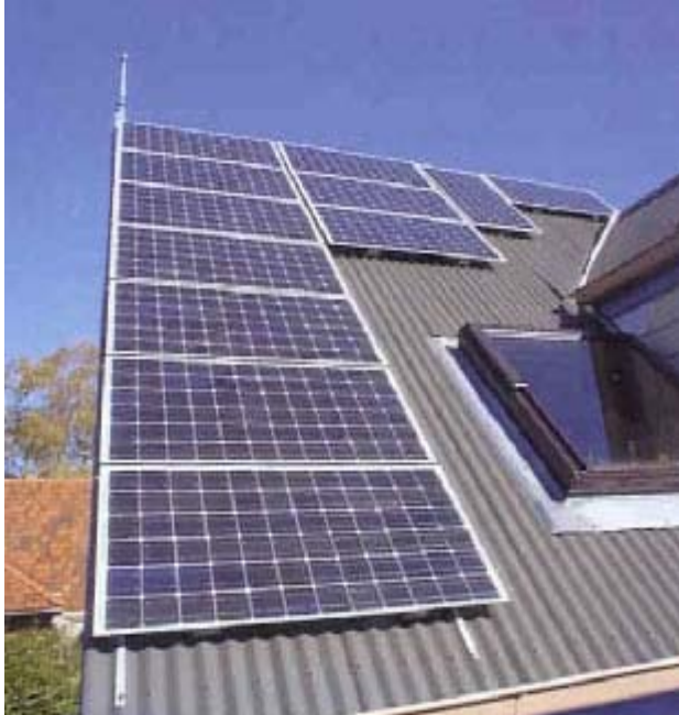
FIGURE 1: ROOF MOUNTED SOLAR INSTALLATION
